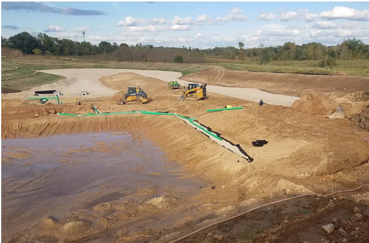
Figure 3: This photo was taken on September 21 st showing the installation of the underdrain collection pipes for the wet pond that connect to the bioretention portion of the pond. Note the stone drainage layer being installed in the bioretention area and the sprouting vegetation on the bioretention area slopes that were seeded earlier in the month.
