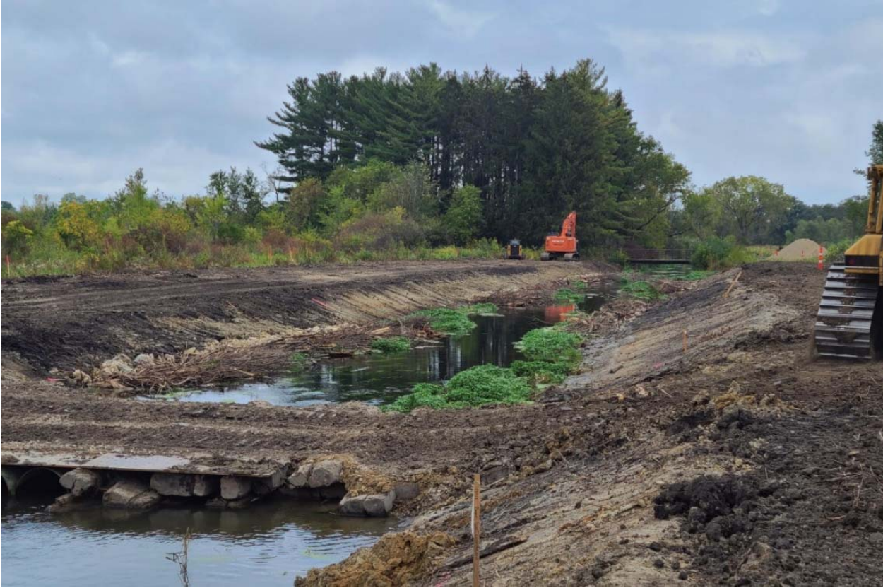
Figure 2: Dane County Streambank Excavation and Log Sills just North of Lincoln Street Channel.
