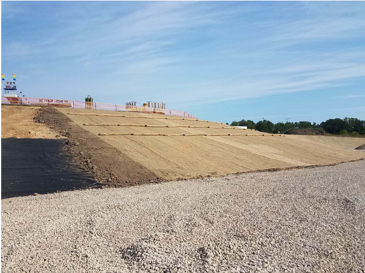
Figure 2: The above photo was taken on September 2 nd showing a portion of the west slope of the bioinfiltration area where the drainage stone has been placed, and the west slope has been topsoiled, seeded, and covered with erosion mat, and erosion logs on the slope installed. A few of the carnival rides associated with Hometown Days are noticeable at the top of the slope behind the construction fence.
