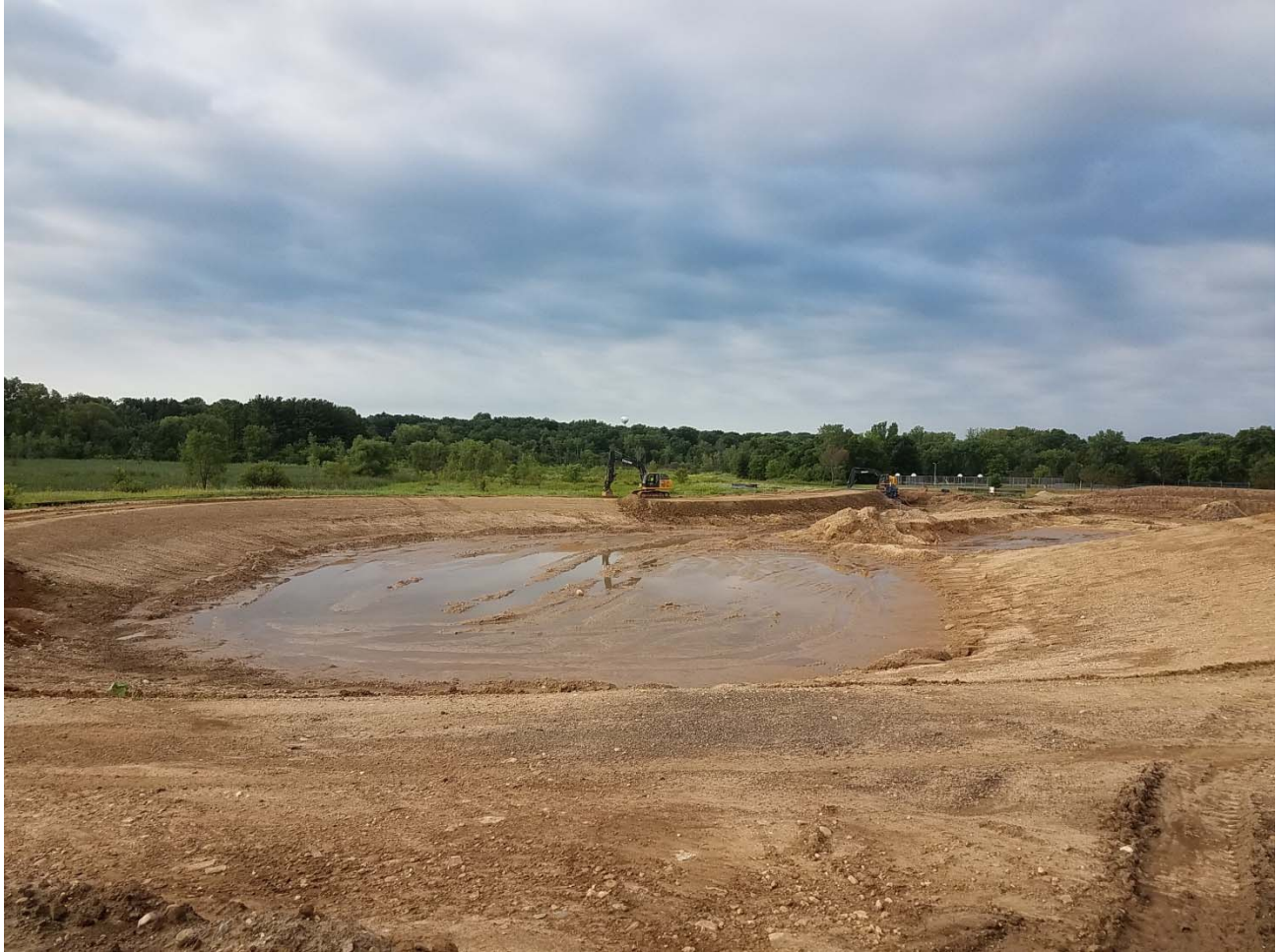
Figure 2: The photo above was taken on July 30th showing the excavation future bioinfiltration area. Note how the berm on the left in the photo is being trimmed back to the design slope.
